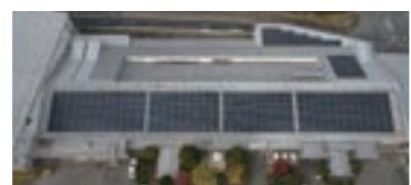
Solar panels at OPC Corporation's Yamanashi Factory (Provided by: The Kansai Electric Power Company, Incorporated)
