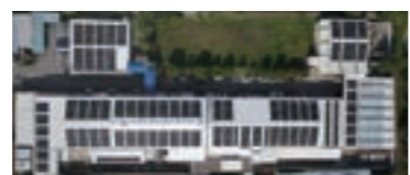
Solar panels at OHARA OPTICAL (M) SDN.BHD. (Malaysia)
