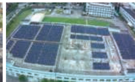
Solar panels installed on roof of OHARA OPTICAL (ZHONGSHAN) LTD. factory
